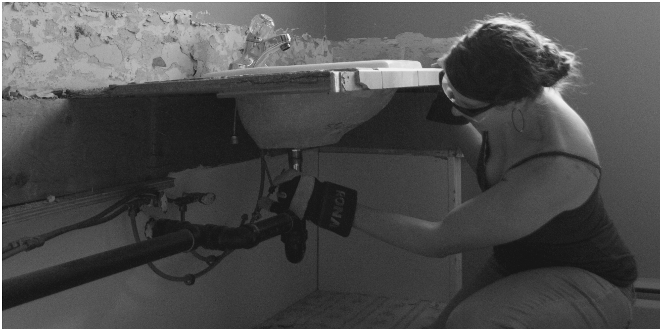
Kristi Hansen is a Red Seal plumber. Calculating the capacity of water lines, determining the length of pipe needed for drainage systems, and accurately predicting the volume of hot water a building's system will use are some of her tasks.
